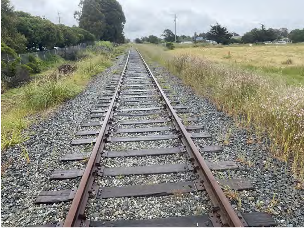
YLR Terrace Photopoint #5 (E). May 3rd, 2023. Photographer: Vaughan Williams Camera: Apple iPad Pro (3rd generation).
